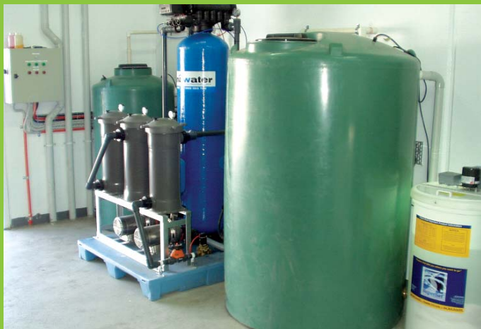
Left: An installation of the water recycling technology developed from the Smart Water Fund research.
