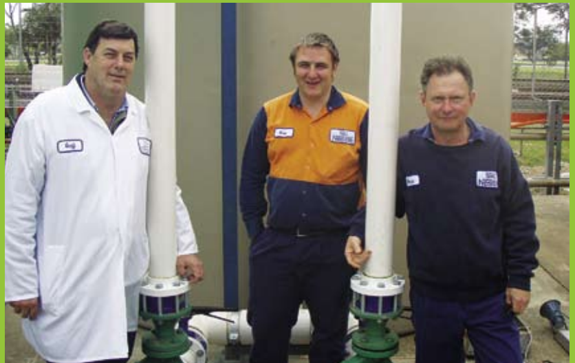
From left, Nestlé's Geoff Young (Project Coordinator), Kris Matlock (Electrical Engineer) and Bruce Warburton (Services Engineer) with their Smart Water Fund rooftop rainwater project equipment. The small transfer water tank is used to feed two larger tanks with a total of 1.2 million litres capacity.
